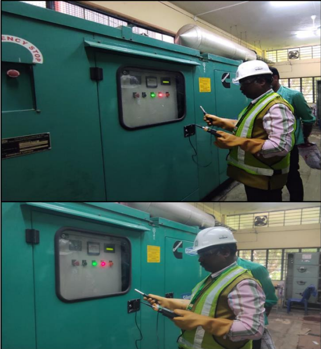
Generator Facility in the JSS College of Arts, Commerce and Science (Autonomous)
